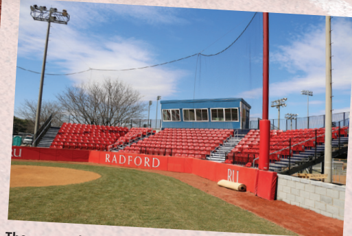
The renovation of Radford Softball's stadium includes new dugouts, stadium seating, a sound system and a press box.
