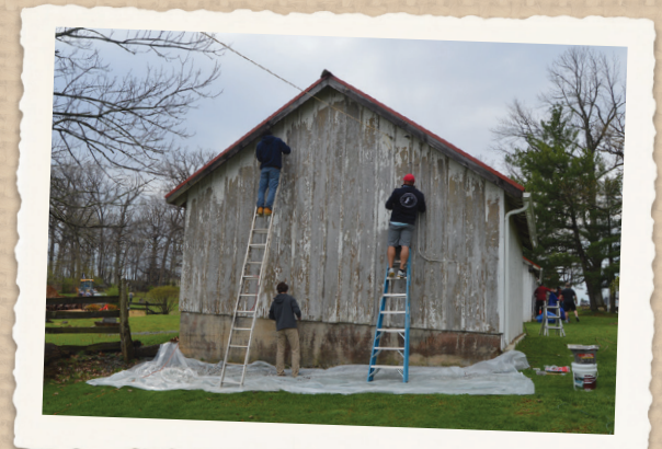
The projects tackled at the Signorello farm included repainting barns, graveling the driveway, cleaning out the pool and repairing fences.
